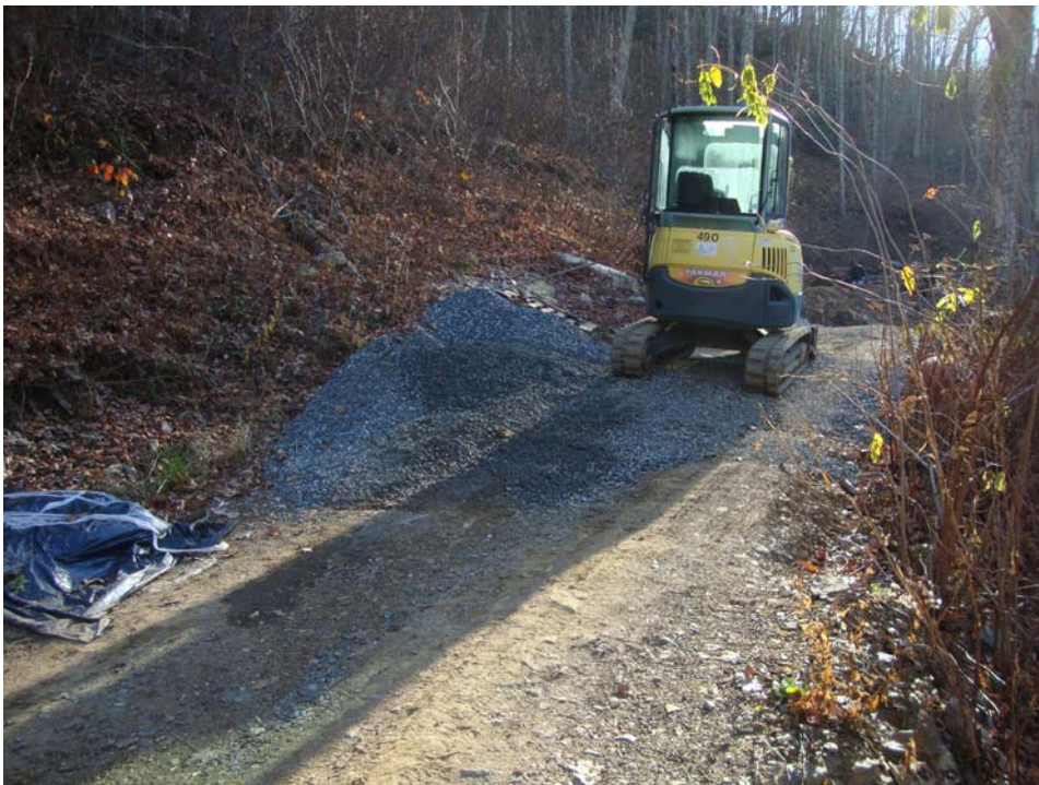
Photo #22: Insured will need to build up driveway in order to bring in (2) 70-ton cranes for recovery.
