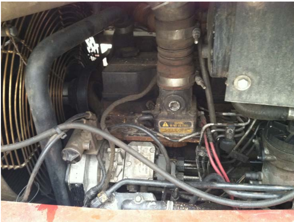
Photo #18: View of Cummins 6-cylinder, ISB series engine. No visible damage to engine.
