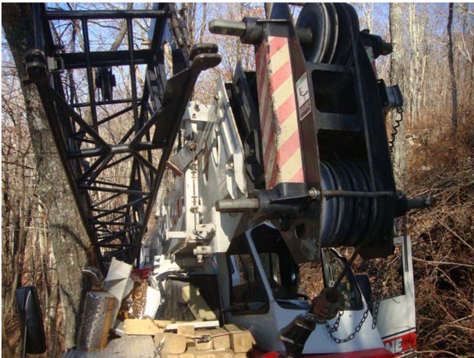
Photo #8: Equipment lodged against tree. Impact damaged jib.
